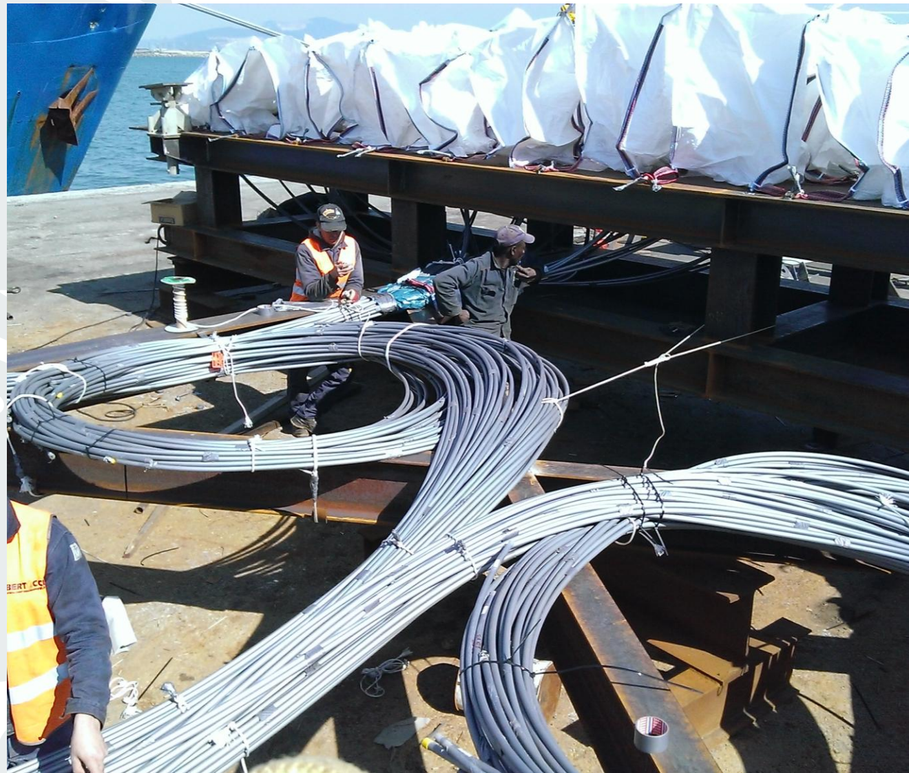
Sireg Geotech high pressure pipes are installed to drive PU resins inside the bags
